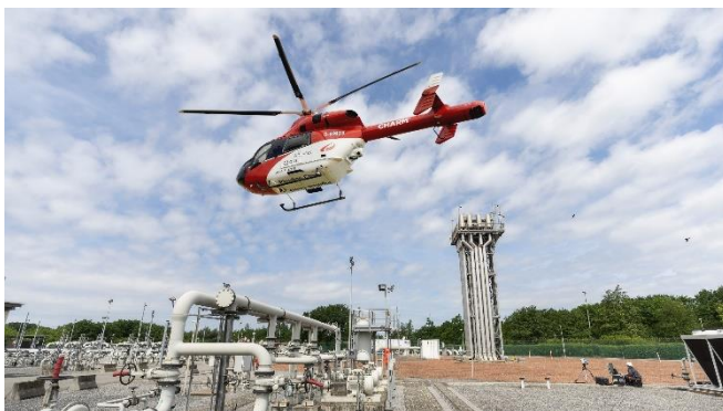
Image 1: The helicopter with the LIDAR system has already flown several 10,000 km and checked pipes for leaks. © Photo Fluxys Belgium - David Samyn.
