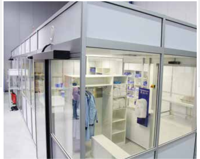
Clean room cell „Hard wall“
