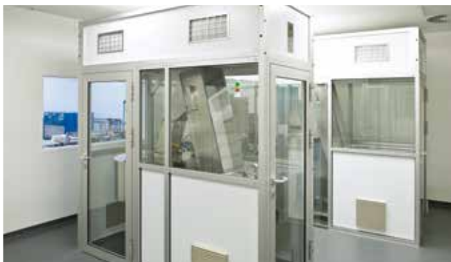
Clean room enclosure of a machine in the pharmacy
